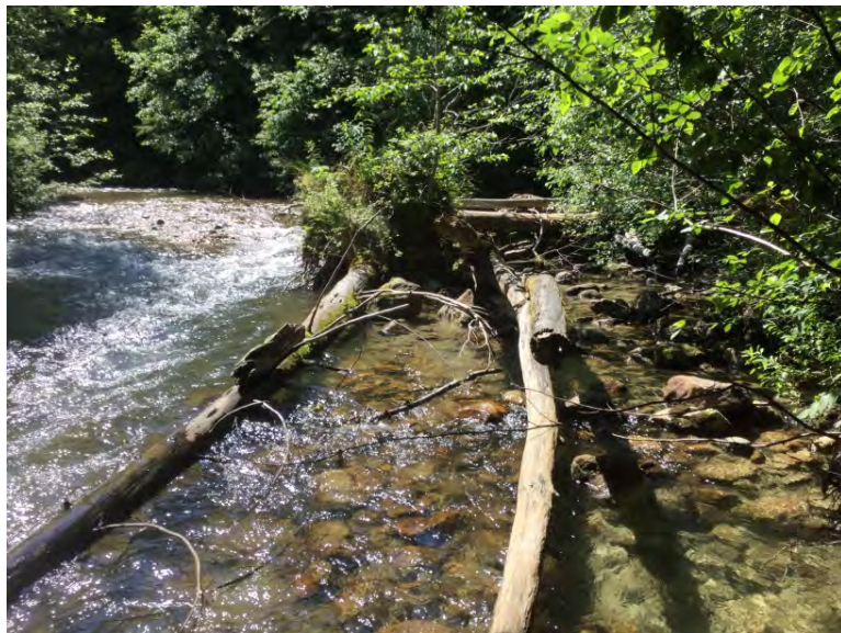
Debris accumulations immediately upstream of crossing
