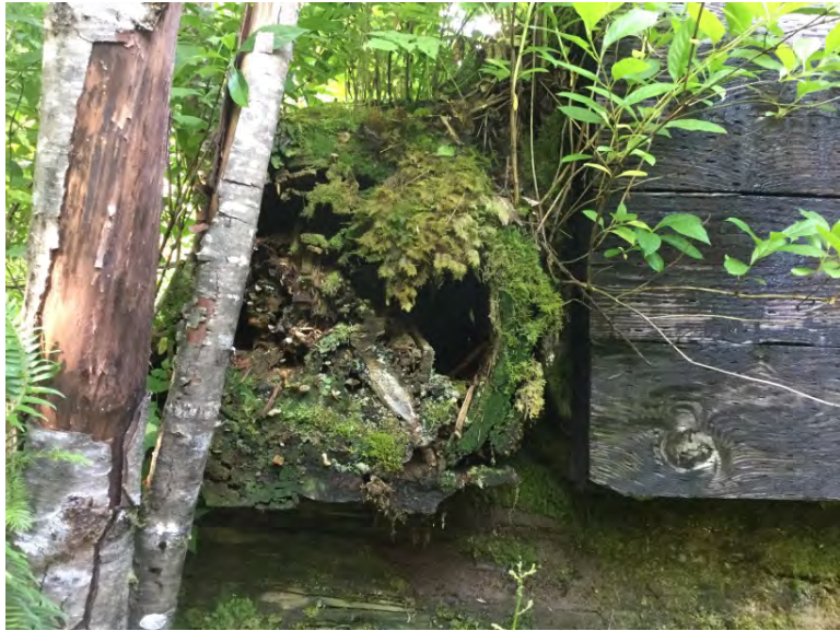
Rotten fill retainment logs at all corners
