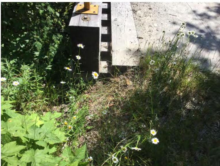
Loosing fill at both approaches
